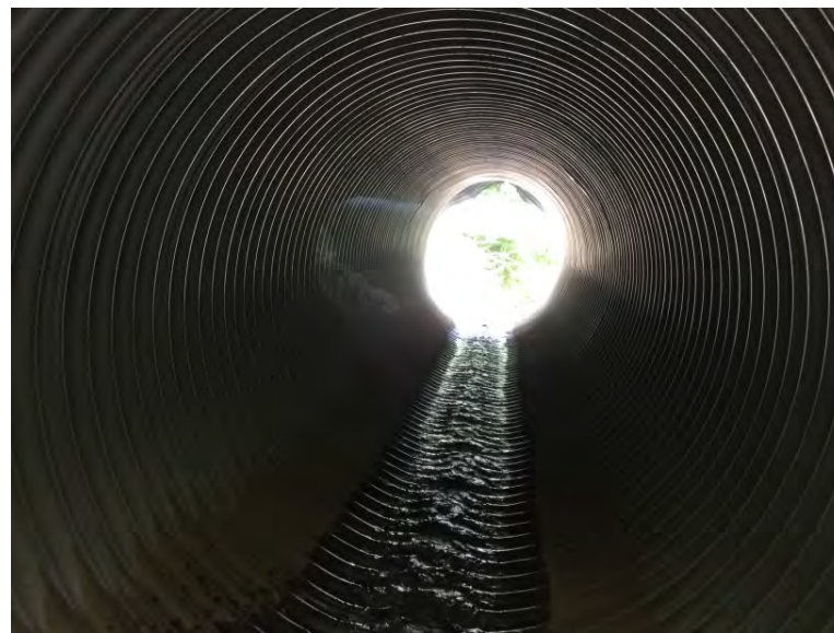
Damage to outlet
