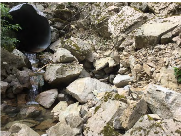
Downstream left bank riprap scour
